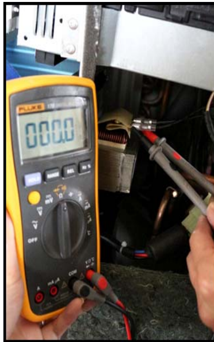
Fig. 19 – Test the Reactor Resistance
