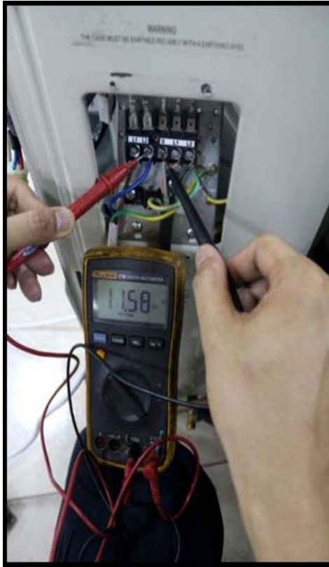
Fig. 18 – Test the DC Voltage
